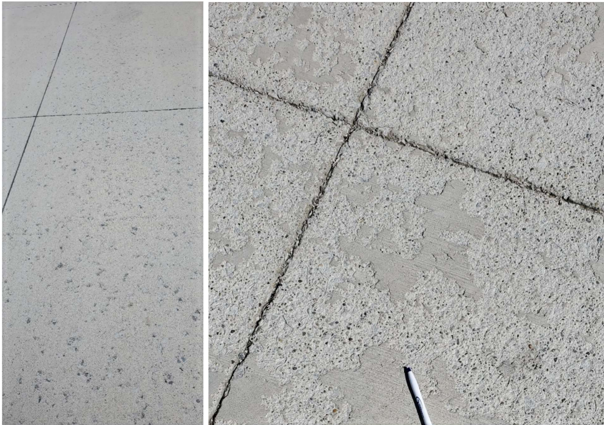
Examples of scaling (left, light severity, sometimes called mortar flaking; and right, medium severity)
