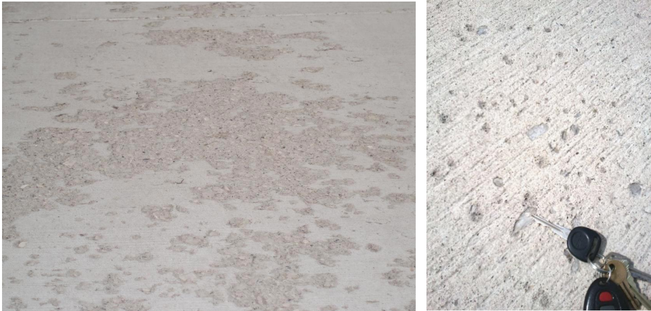
Examples of scaling (left, medium severity; and right, light severity, sometimes called mortar flaking)
